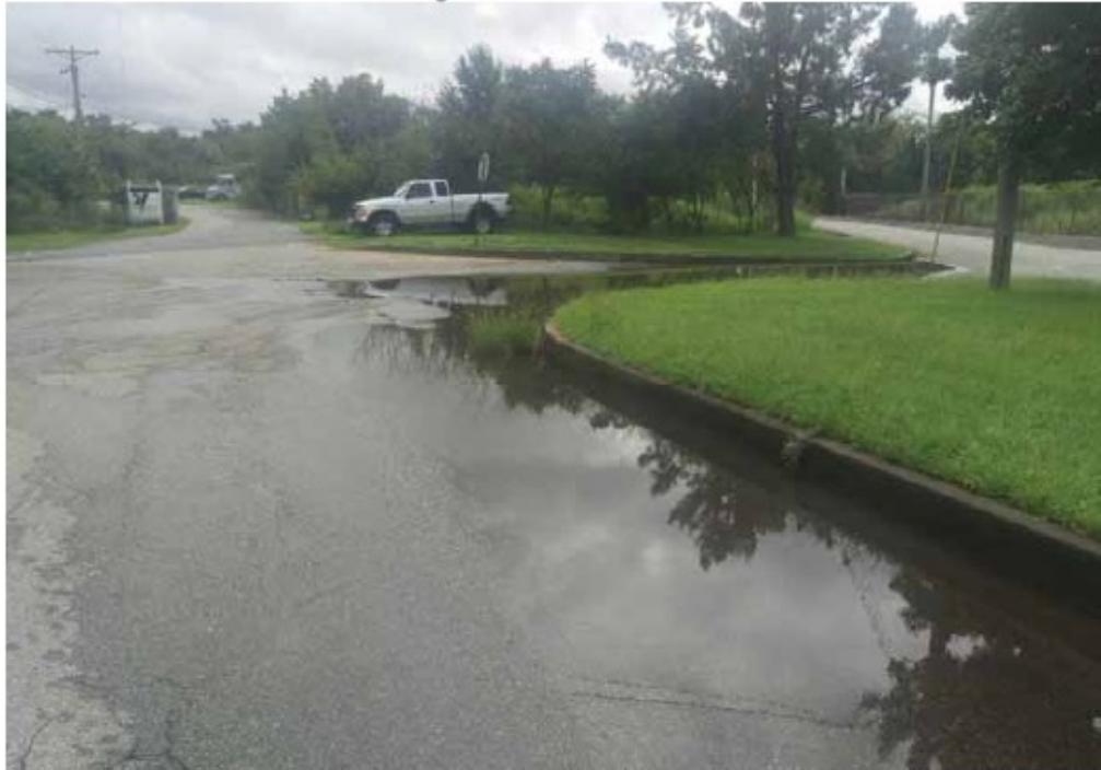
Figure 1: A photograph of the submerged intersection of 7th Street and Industrial Ave.
