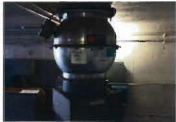
Loren Cook Ventilation Fan High Temperature exhaust Model: 10CV17D 20 A Breaker, 115 V; 1725 RPM; 1/6 HP S/N: 289S647944000007010601
