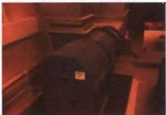
Exhaust Fan - EF-1 Twin City Corporation - No Data Available Two motor dampner Location: Pump Room Belt: 4L-330
