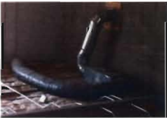
Electric Vent fan in office near Maintenance Shop No Data Maintenance Supervisor Office in Smoke Stack Building
