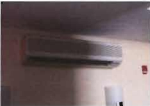
Staircase Split Unit
