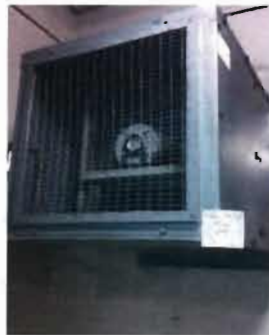
Exhaust Fan - EF-1 Location: Pump Room Greenheck Model No. SE2-16-417-A3 Serial No: 06100123 Direct Drive
