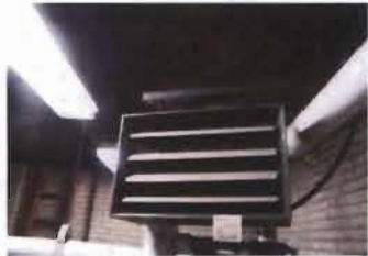
Locker Area Near Boiler Trane Steam Unit Heater Model No UHSA-038S-8C-AAC S/N: D91H08892
