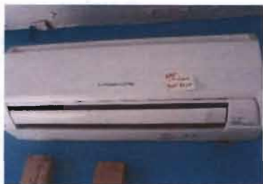
Mitsubishi Electric Heat Pump, Split System Model No MSZ-A17NA Serial No. 6003457-T 208 V; 1 Phase Location: 2nd Floor Shop Area
