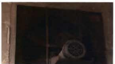
Non functional Fan and Louver Electrical Store Room To be cleaned annually
