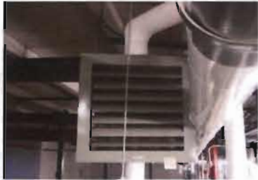
Hydronic Unit Heater Modine Model No. HSB193SB01SA (Year: 2018) Serial No. 43104417-2301 1/3 Hp; 115 V; 4.2 Amp Near Sed Basin No 3 South Side
