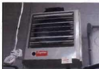
Lime Silo - Upper Dayton Unit Heater Model No. 2YU70 480 V; 10 KW; 3 Phase; 0.22 Amp
