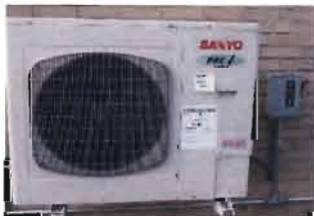
Split Unit on Roof Sanyo R410A Model C3672R S/N: 0015111 230 V; 13.8 Amp; single phase
