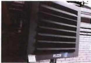
Steam Unit Heater Modine Hydronic Unit Heater Model No. HSB165S01 S/N: 30104407-3969 1/3 Hp; 115 V, 4.6 Amp Location: Basement Near Old Pump 3A/3B
