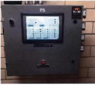
Control Panel for VFD Controlled Exhaust Air EF-1, -2 and -3
