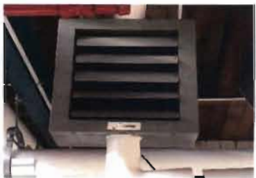
Hydronic Unit Heater Modine Model No. HSB 86S01 Serial No. 38014208-2683 1/8 Hp; 115 Volt; 2.3 Amps Location: Near Meter Shop
