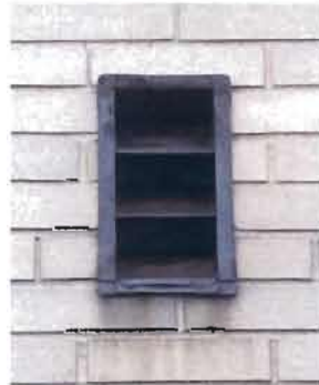
Outside Louver Associated with Men's Room Fan Clean annually
