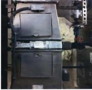
Duct Heater Heat Exchanger Trane Coil Type: NS Sigma Flo Serial No. H12E04662 Order No. D2T823A Serv. Model No. DNSB12016GOAA064AADA00B0000 Coil Serial No. 122012060B Location: Membrane floor, above air compressors - (Photograph view from above)
