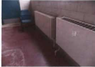
Break Room Four (4) Steam Radiators No Data
