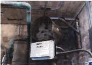
Screen House - Chromalox Electric Unit Heater Cat No. HD3D-500 S/N: 004-305492-010 240 V; 5 KW; 1 Phase
