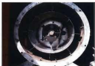
View inside Exhaust Fan Enclosures No Data available Direct Drive
