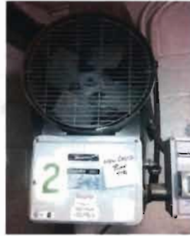
Electric Unit Heater - EUH-2 Location: Pump Room Chromoloz Model No. HD3D-750 Serial No. 004-305492-023 480 V; 7.5 KW; 3 Phase
