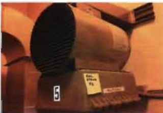
Electric Unit Heater - EUH-5 Marley Electric Heater Model No. W50041A Corrosion Resistant/Washdown MFG Code - L94 5 KW; 240 V; Single Phase Location: Pump Station
