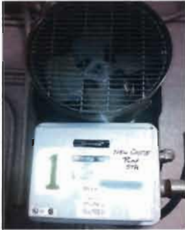
Electric Unit Heater - EUH-1 Location: Pump Room Chromoloz Model No. HD3D-750 Serial No. 004-305492-023 480 V; 7.5 KW; 3 Phase
