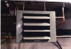
One Hydronic Unit Heat in basement of Gate House Modine Model No. 47SB01SA Serial No. 39105018-5464 1/12 Hp; 115 volt; 1.7 Amp
