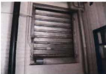
Motorized Louver 24" x 40" No Data Near Meter Shop
