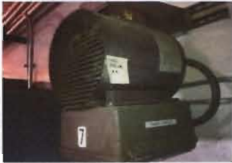
Electric Unit Heater - EUH-7 Marley Electric Heater Model No. W50041A Corrosion Resistent/Washdown MFG Code - L94 5 KW; 240 V; Single Phase Location: Pump Station
