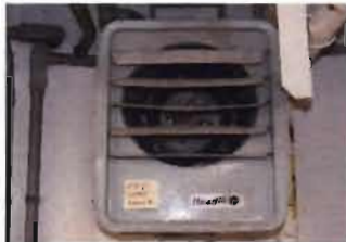
Lime Silo - Lower Heatflo Unit Heater - Electric No Data
