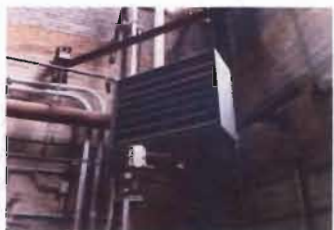
Steam Unit Heater Trane Model UHSA 126S-8C-AAF Type 136-109-01 S/N: D85G00902 Location: Boiler Room
