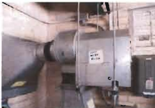
Metering Building Greenheck Blower Fan, Ducted Model No. SFD-S-SB-C4-TH S/N: D4H23929 EF-1 Direct Drive
