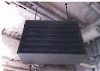
Steam Unit Heater Trane Model UHSA 10058AAAE Type 136-108-01 S/N: D82K4571 Location: BPS Basement near Old Pump 3A/3B
