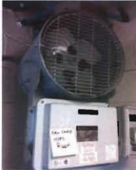
Electric Unit Heater - EUH-3 Location: Hypo Room Chromolox Model No. HD3D-500PS Serial No. 004-305708-120 480 V; 5 KW; 3 Phase
