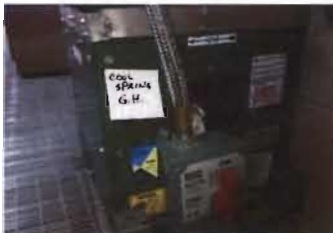
Exhaust Fan - EF-4 ILG Model No. 5508.SQDA08E16 Serial No. 081007M287820 Location: Cool Spring Gate House Direct Drive
