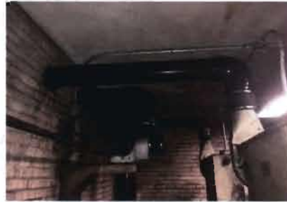
Carbon Room ductwork to be cleaned Annually
