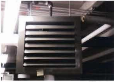
Hydronic Unit Heater Modine Model No. HSB193SB01SA (Year: 2018) Serial No. 43104517-1191 1/3 Hp; 115 V; 4.2 Amp Location: No. 8 Sed Basin - north
