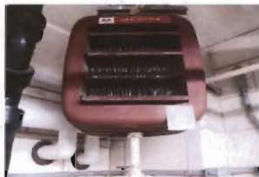
Steam Unit Heater Modine Model No. HS33501 Serial No. SP0011996 Location: ACH Feed Room
