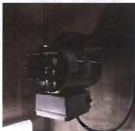
Metering Building Unit Heater Marley Electric Washdown/Corrosion Resistant Model No. QWD 05212BT000 5.0 KW; 240 V; 1 Phase; 22.6 Amp Installed in January 2017
