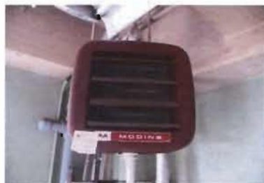
Steam Unit Heater Modine Model No. HS33S01 Serial No. SP011996 Location: Old Generator Room
