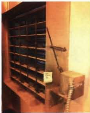
Damper No. 6 Motorized Wall Unit Location: Pump Room
