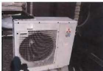
BMP - Rooftop Units Mitsubishi R410A, Mr. Slim Split Unit Matches to Foreman's Office Model MXZ-3A30NA 208/230 V; 1 Phase S/N: 61901162B
