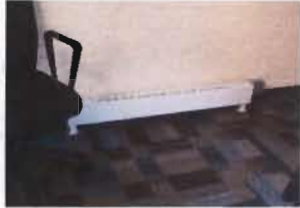
Conference Room First Floor Floor Radiator
