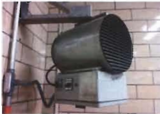
Markel Electric Unit Heater Quantity: 3 Model: F3F5505T 208 Volt; 5 KW; 3 Phase; 0.7 Amp
