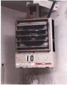
Dayton Electric Unit Heater 240 V; 3.3 KW Location: Former Chlorine Room in Pump Station
