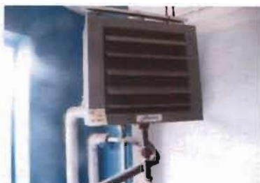
Hydronic Unit Heater Modine Model No HSB86501 Serial No. 38014008-1638 1/8 Hp; 115 V; 1 Phase; 2.3 Amp Shop Area - 2nd Floor
