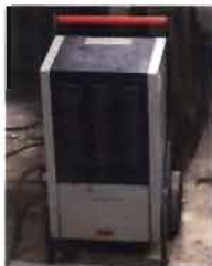
Dayton Dehumidifier Unit Located in Basement of Gate House
