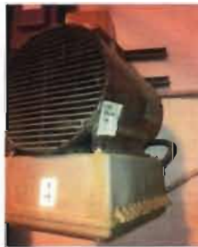
Electric Unit Heater - EUH-4 Marley Electric Heater Model No. W75041A MFG Code - L94 7.5 KW; 240 V; Single Phase Location: Pump Station
