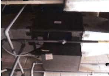
Ventilator Penn Model SX125BC Location: Hypo Room
