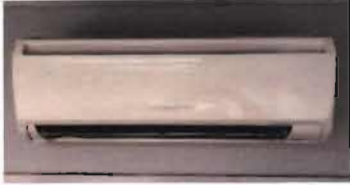
Mitsubishi Split System Heat Pump Model No. MSZ-A09NA Serial No. 6003970 208/240 V; Single Phase Maintenance Supervisor Office in Smoke Stack Building
