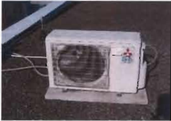
BMP - Rooftop Units Mitsubishi R410A, Mr. Slim Split Unit Matches to Meter Shop Office Model MUZ-09NA 208/230 V; 1 Phase S/N: 6003328
