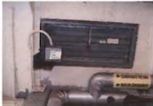
PFP - Hypo Room Motorized Louver No Data
