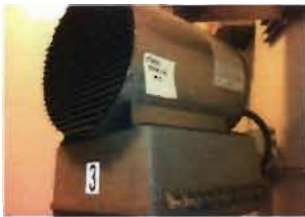
Electric Unit Heater - EUH-3 Marley Electric Heater Model No. W75041A MFG Code - L94 7.5 KW; 240 V; Single Phase Location: Pump Station
