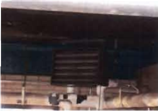
PFP - Garage Trane Steam Unit Heater Model No UHSA-060S-8C-AAE S/N: D91H08897
