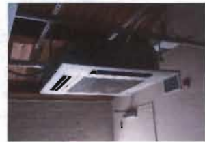
Second Floor Conference Room Split Unit
