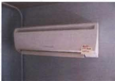
Mitsubishi Heat Pump, Split System Model No. MSZ-A12NA Serial No. 6004080-T 208 V; 1 Phase Location: Foreman's Office
