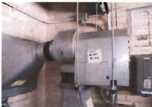
Metering Building Greenheck Blower Fan, Ducted Model No. SFD-S-SB-C4-TH S/N: D4H23929 EF-1 Direct Drive
