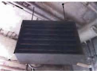
Steam Unit Heater Trane Model UHSA 10058AAAE Type 136-108-01 S/N: D82K4571 Location: BPS Basement near Old Pump 3A/3B
