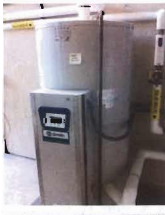
Automatic Electric Water Heater AO Smith Model DSE120A Serial No. 1301R000001 Item ID: 9500010810 120 Gals; 3 phase; 480 V; 7 Amp; 6000 Watt Location: In Membrane Area
