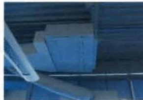
Cubicle Area Ventilation Units
