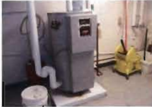
Water Heater Bradford White Model No, MII5093SF09 S/N: FC11755636 50 Gallons; 9 KW
