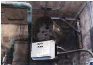
Screen House - Chromalox Electric Unit Heater Cat No. HD3D-500 S/N: 004-305492-010 240 V; 5 KW; 1 Phase
