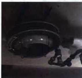
PFP - Basement Modine Steam Unit Heater Unit No. V59SB01SA S/N: 39013616-5261 115 V; 1 Phase; 1.4 A Replaced in 2017 Near Stairs
