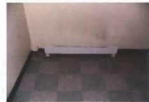
Basement Staircase Floor Radiator
