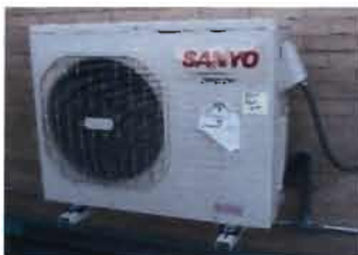
Split Unit on Roof Sanyo R410A Model C2472 S/N: 0044012 85221344675000 230 V; 10.8 Amp; single phase Date: 4/11
