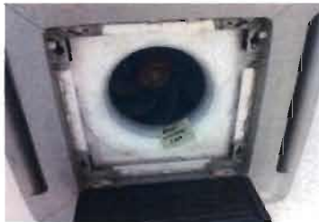
EMI Ductless Series Split Unit Model No. S1HG2000D12 Serial No. 1-12-F-6919-24 208/240 V; Single Phase Location: Control Room
