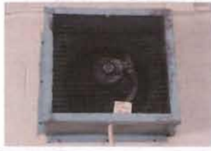
PFP - Fluoride Room 18-inch Exhaust Fan No Data
