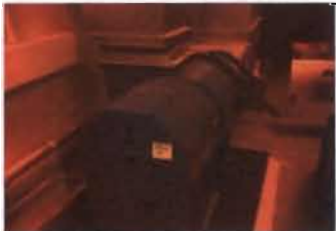
Exhaust Fan - EF-1 Twin City Corporation - No Data Available Two motor dampner Location: Pump Room Belt: 4L-330
