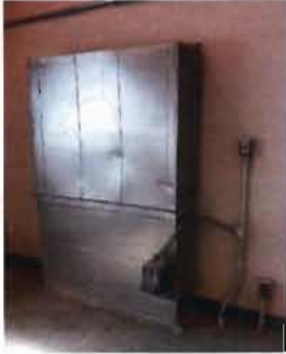
Damper No. 2 and 3 Motorized Wall Unit Ducted to Basement Location: Pump Room
