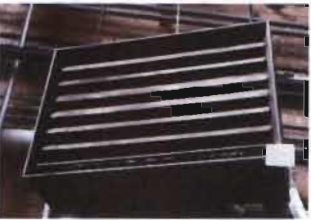
Steam Unit Heater Trane Model UHSA 12658AAAE Type 136-109-01 S/N: D83M03888 Location: Boiler Room
