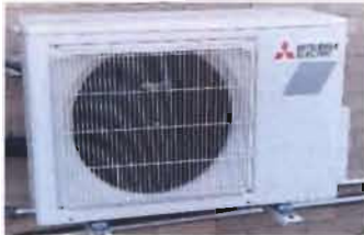
Split Unit on Roof Mitsubishi Model MUZ-FH09NA 230 V; 15 Amp R410A Refrigerant
