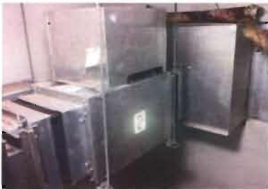
Exhaust Fan EF-2 Location: Pump Room Greenheck Model No. BSQ-80-3 Serial No. 06H26880 Belt: 4L-370R Includes intake louvers
