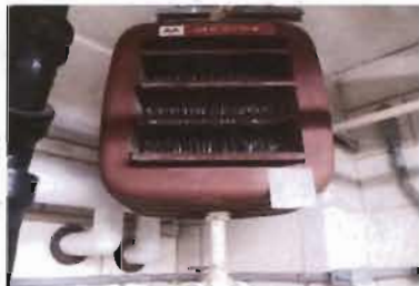
Steam Unit Heater Modine Model No. HS33501 Serial No. SP0011996 Location: ACH Feed Room
