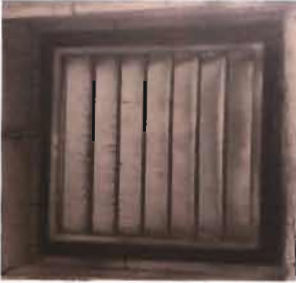
Interior louvers to be cleaned annually
