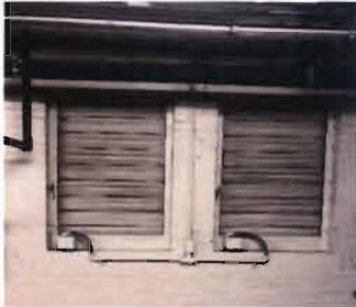
Motorized Louvers - 40" x 30" No Data Near Sed Basin No. 1
