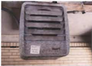
PFP - Sludge Building Heatflo Unit Heater - Electric Cat No. HLH-C-10-43-30-00 MFG Part No. 004-303380-503 10 KW; 480 V
