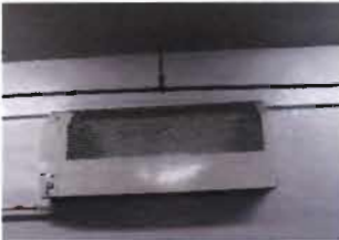
Chromalox Electric Unit Heater Cat No. HCH-501M 277 V; 1 Phase; 5000 Watts EF-7 - Lower Level Pump Area
