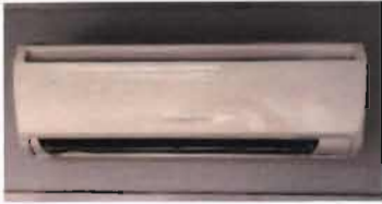
Mitsubishi Split System Heat Pump Model No. MSZ-A09NA Serial No. 6003970 208/240 V; Single Phase Maintenance Supervisor Office in Smoke Stack Building
