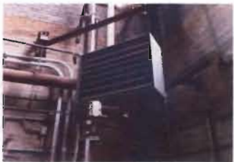
Steam Unit Heater Trane Model UHSA 126S-8C-AAF Type 136-109-01 S/N: D85G00902 Location: Boiler Room
