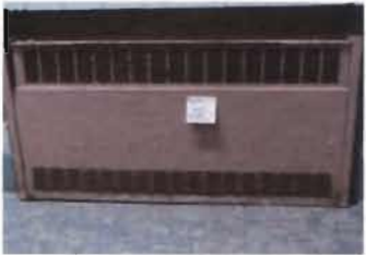
Men's Rest Room Wall Unit - Steam Radiator No Data
