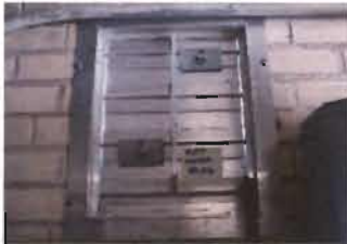
Metering Building Gravity Damper - One No Data
