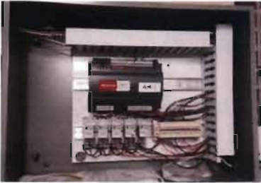
Honeywell Spyder Sylk Enhanced Air Handler Controller AH-1 Location: Electrical Room
