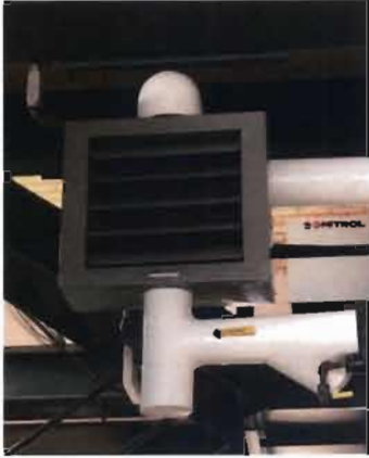
Modine Hydronic Unit Heater Model: HSB 86SB01SA S/N: 39011019-5335- 1/8 Hp, 115V 2.2 Amps Typical of four on Third Floor Washwater Tank Area
