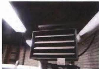
Locker Area Near Boiler Trane Steam Unit Heater Model No UHSA-038S-8C-AAC S/N: D91H08892
