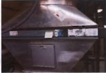
Duct Heat Exchanger - 24" x 42" Steam Trane Coil Type NS Sigma Flo Serial No. H12E04661 Order No. D2T823A B/L A Air from a roof top unit Location: Near rear entrance
