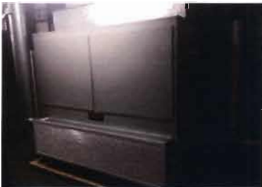
Trane Electric Heater Model: TWE180E300AA Serial No: 12204XCYWA Date: 5/20/12 Location: Electrical Room
