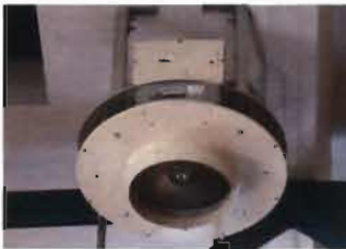
Chromalox Electric Unit Heater Main Floor Ceiling 277 V; 1 Phase VUH-2
