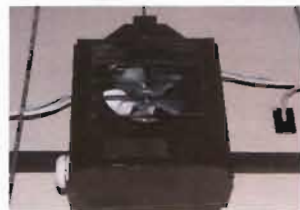
Utility Room Second Floor Berko Unit Heater
