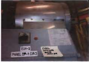
Electric Unit Heater - EUH-3 Location: Cool Spring Gate House TPI Corporation Model No. P3P5515 43WD1501 480 V; 15 KW; 3 phase
