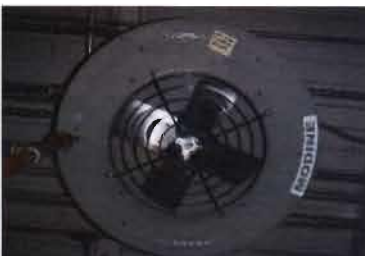
Modine Steam Unit Heater Model No. V139SB06SA Serial No. 18014017-5060 (Year: 2018) 1/6 Hp; 115 Volt, 2.3 Amp Location: Hallway near Carbon Room
