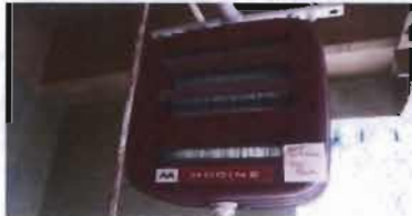
Steam Unit Heater Modine Model HS47S01 Serial No. SP011996 Location: Tool Room
