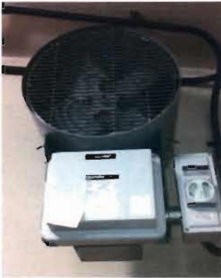
Electric Unit Heater - EUH-1 Chromolox Model No. HD3D-1000PST 004-305709-089 480 V; 10 KW; 3 Phase Location: Hypo Room
