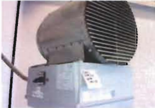
Electric Unit Heater - EUH-4 Location: Cool Spring Gate House TPI Corporation Model No. P3P5515 43WD1501 480 V; 15 KW; 3 phase
