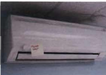
Mitsubishi Heat Pump Split System Model MSZ-A09 NA Serial No. 6003579 208 V; 1 Single Location: Meter Shop
