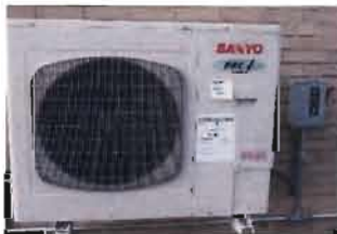
Split Unit on Roof Sanyo R410A Model C3672R S/N: 0015111 230 V; 13.8 Amp; single phase
