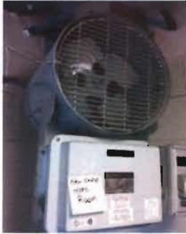
Electric Unit Heater - EUH-3 Location: Hypo Room Chromolox Model No. HD3D-500PS Serial No. 004-305708-120 480 V; 5 KW; 3 Phase
