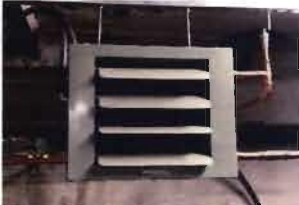
One Hydronic Unit Heat in basement of Gate House Modine Model No. 47SB01SA Serial No. 39105018-5464 1/12 Hp; 115 volt; 1.7 Amp
