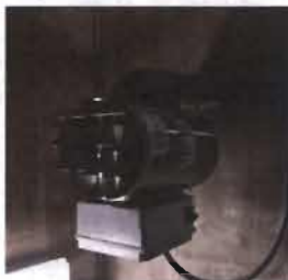
Metering Building Unit Heater Marley Electric Washdown/Corrosion Resistant Model No. QWD 05212BT000 5.0 KW; 240 V; 1 Phase; 22.6 Amp Installed in January 2017
