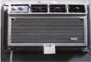
Whirlpool Air Conditioner Window Unit Location: Pump Station, Supervisor Office
